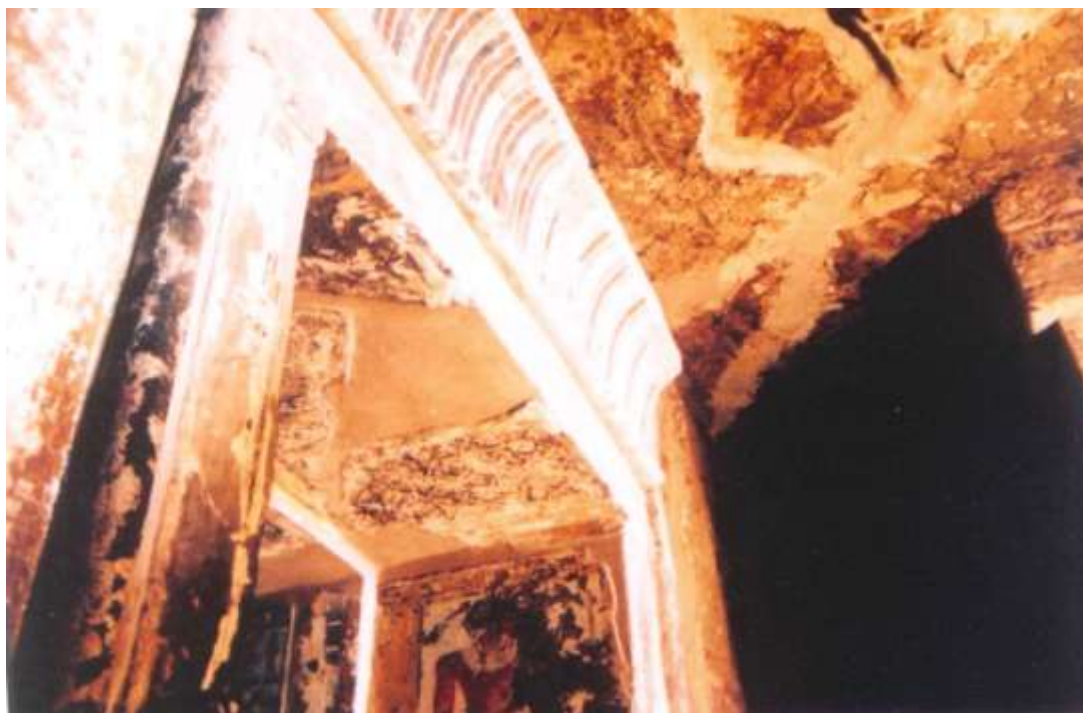
Fig. 3 Deterioration inside one of the Elephantine tombs.
